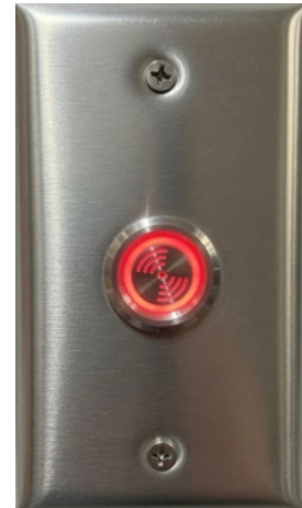
Inside Light / Alarm
